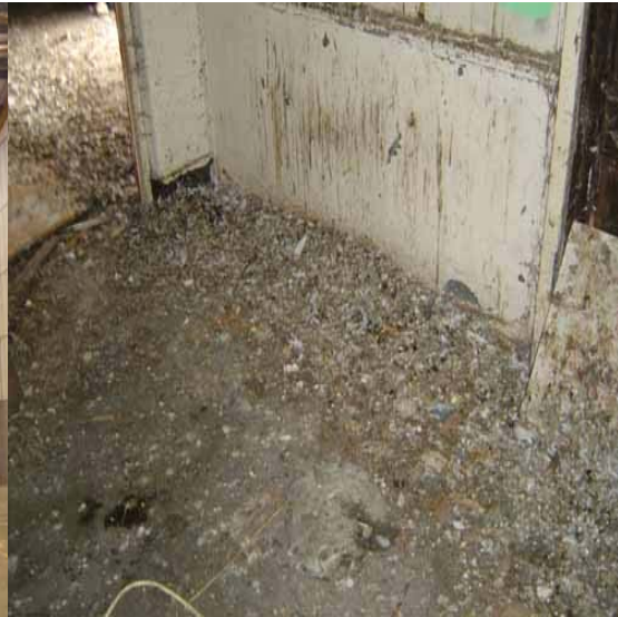
Pigeon Droppings Treated & Cleared
